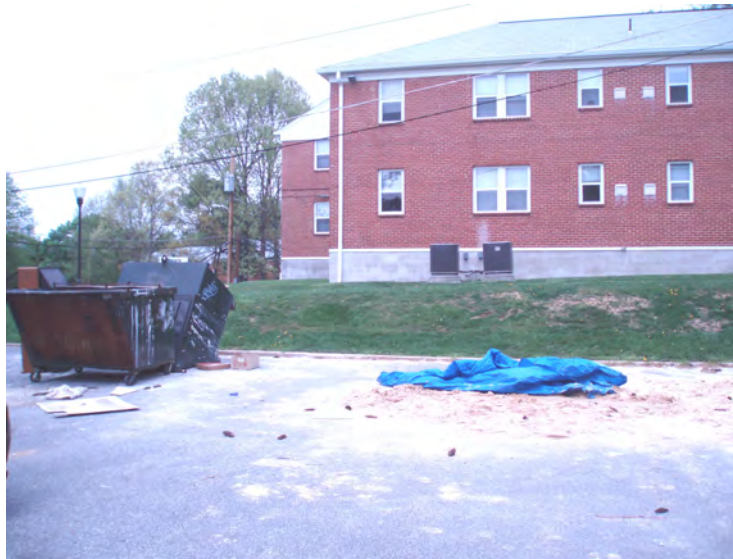
poor sediment control in NSA-L-89
