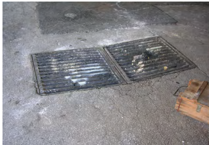
evidence of paint dumping at ISI-L-154
