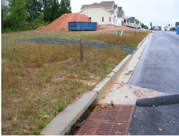
poor sediment control in NSA-L-177
